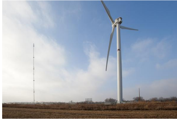
Figure 1. Clipper Liberty C96 2.5 MW wind turbine at University of Minnesota [34].
