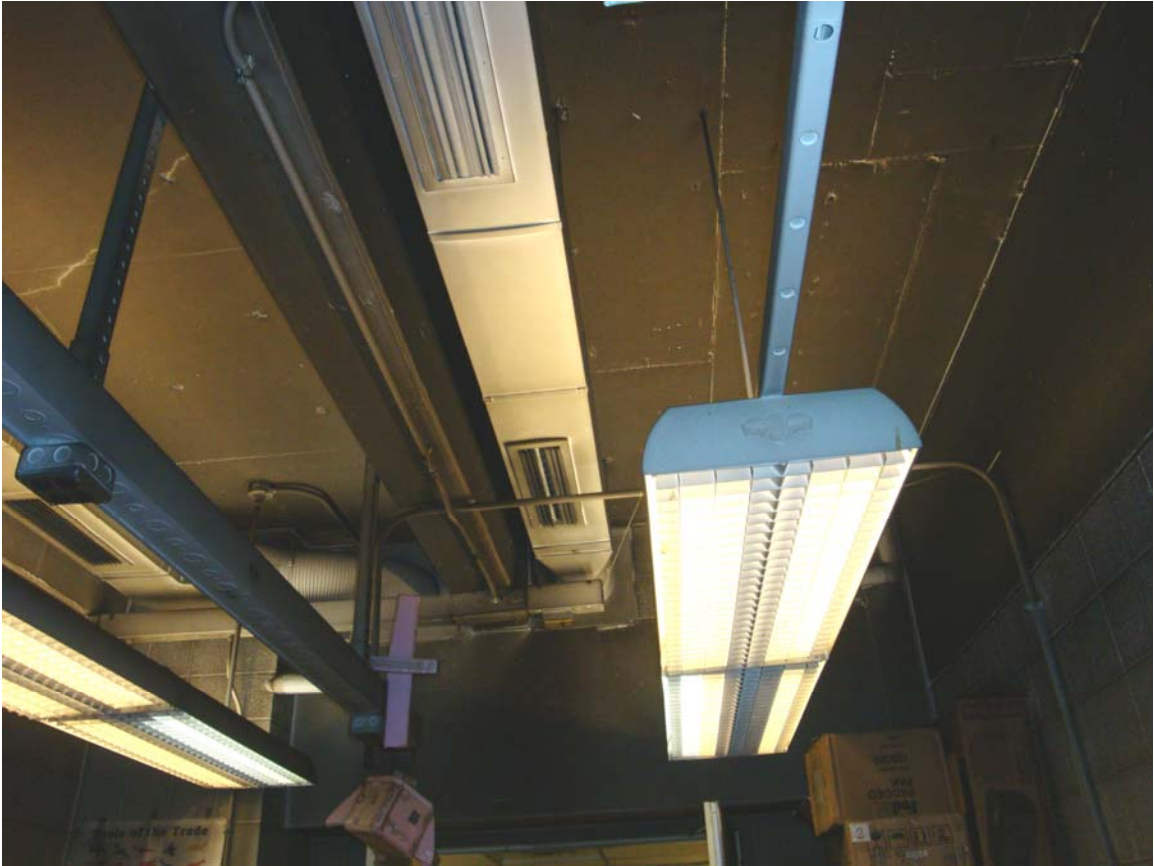
Soot on the ceiling
