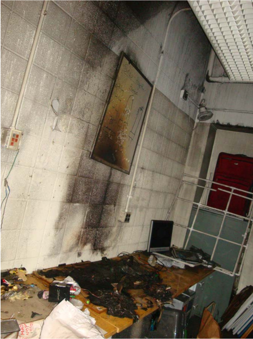
Fire and smoke source
